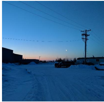
Existing mine site power distribution infrastructure
