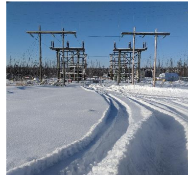
Manitoba Hydro substation at Sherridon Manitoba
