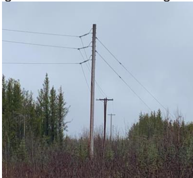
Power line infrastructure to be purchased from Manitoba Hydro
